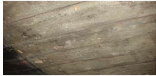
Rare wood ceiling in current kitchen. Identification assistance from photos sent to Department of Historical Resources, Virginia and U.S. Department of Forestry. Preservation by both entities was suggested.
