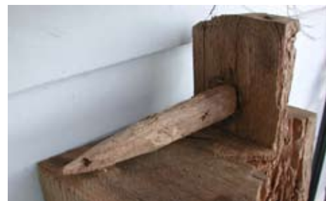
Pegged sill section removed during east/front sill replacement. Note difference in style from rear pegged sill (above).
